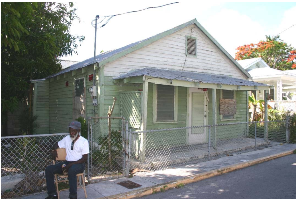
Top Photograph: Vehicles Parked in Yard, Amelia Street (Source: City of Key West, 2009); Bottom Photograph: Deteriorated House, Virginia Street (Source: City of Key West, 2009)
