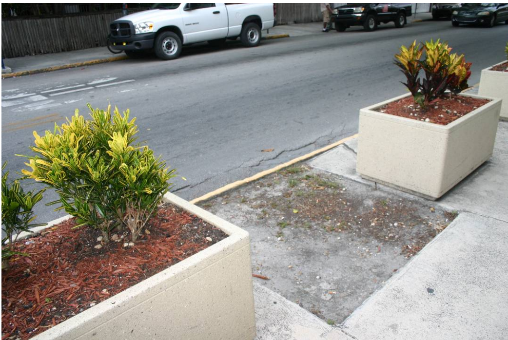
Top Photograph: Deteriorated Sidewalk, Caroline and Simonton Street (Source: City of Key West, 2009) Bottom Photograph: Deteriorated Fence, Caroline Street (Source: City of Key West, 2009)
