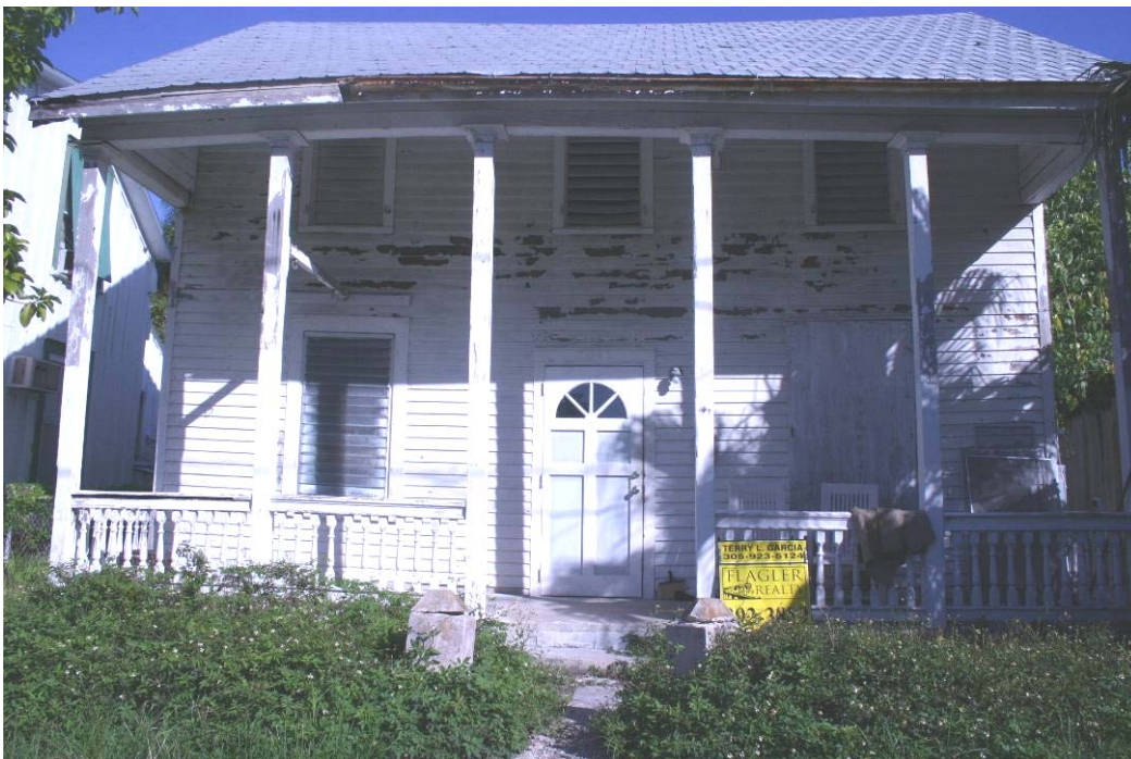
Top Photograph: Deteriorated Building, James Street (Source: City of Key West, 2009); Bottom Photograph: Deteriorated House, James Street (Source: City of Key West, 2009)
