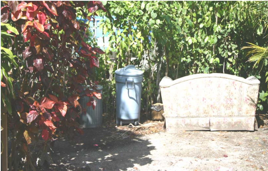
Top Photograph: Broken Concrete Block Wall (Source: City of Key West, 2009); Bottom Photograph: Abandoned Furniture, Mickens Lane (Source: City of Key West, 2009)
