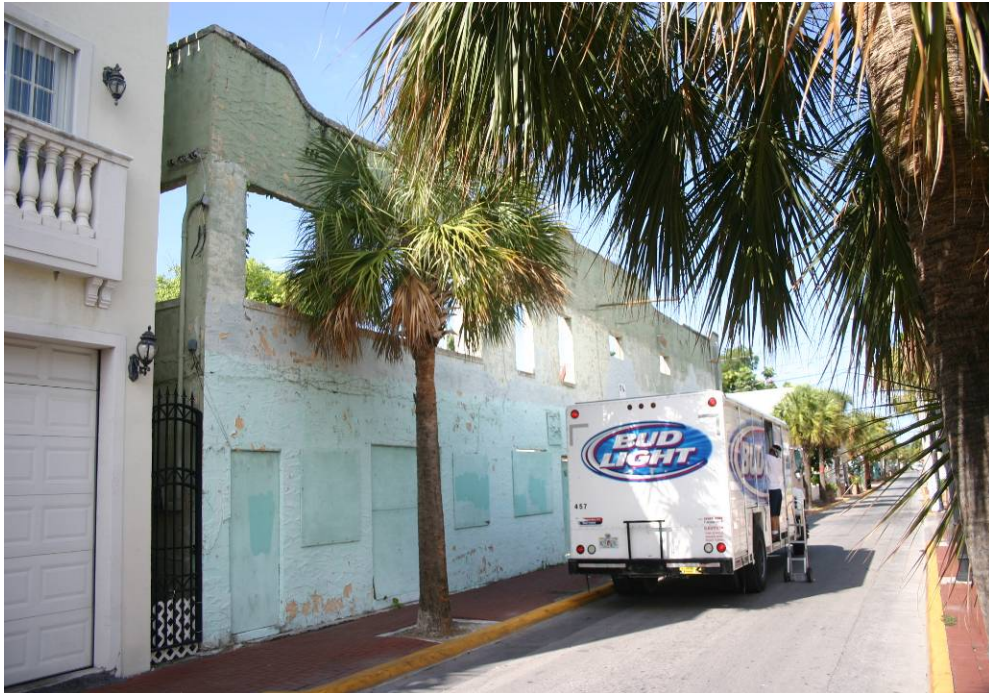
Top Photograph: Entrance to Bahama Village, Petronia and Duval Street (Source: City of Key West, 2009); Bottom Photograph: Dilapidated Building, Petronia Street (Source: City of Key West, 2009)
