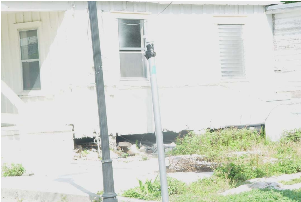
Top Photograph: Vacant Commercial, Petronia Street (Source: City of Key West, 2009) Bottom Photograph: Deteriorated House, Petronia Street (Source: City of Key West, 2009)
