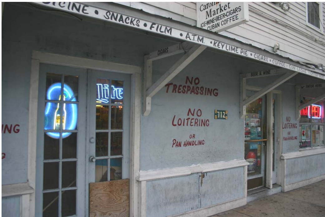
Top Photograph: Deteriorated House, Caroline Street (Source: City of Key West, 2009)
