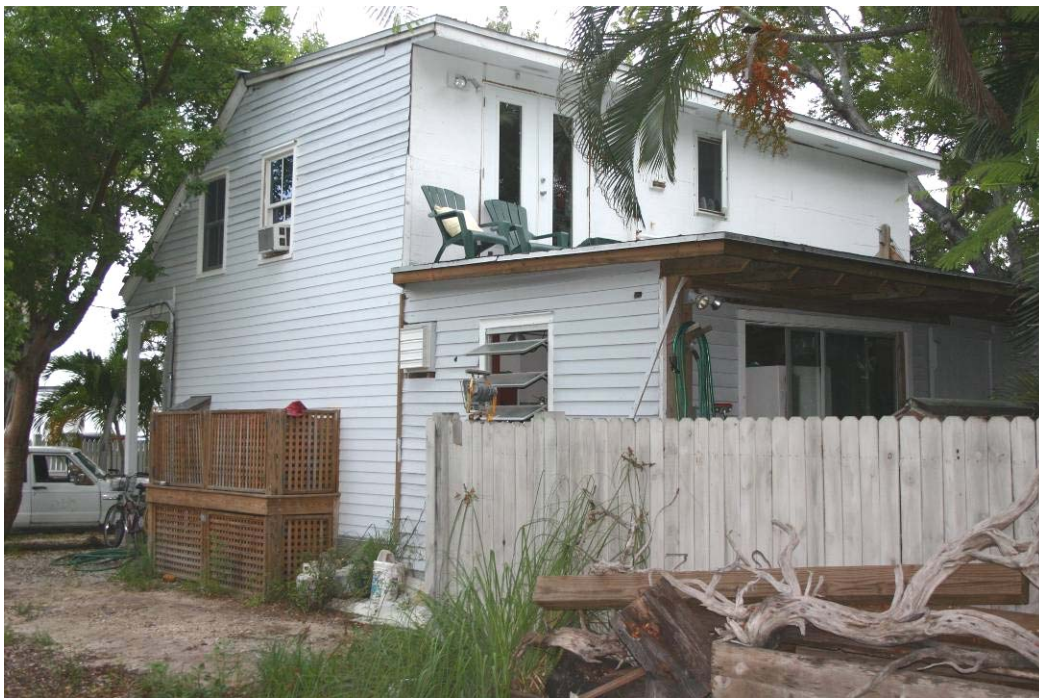
Top Photograph: Deteriorated House, William Street (Source: City of Key West, 2009); Bottom Photograph: Deteriorated House, William Street Area (Source: City of Key West, 2009)
