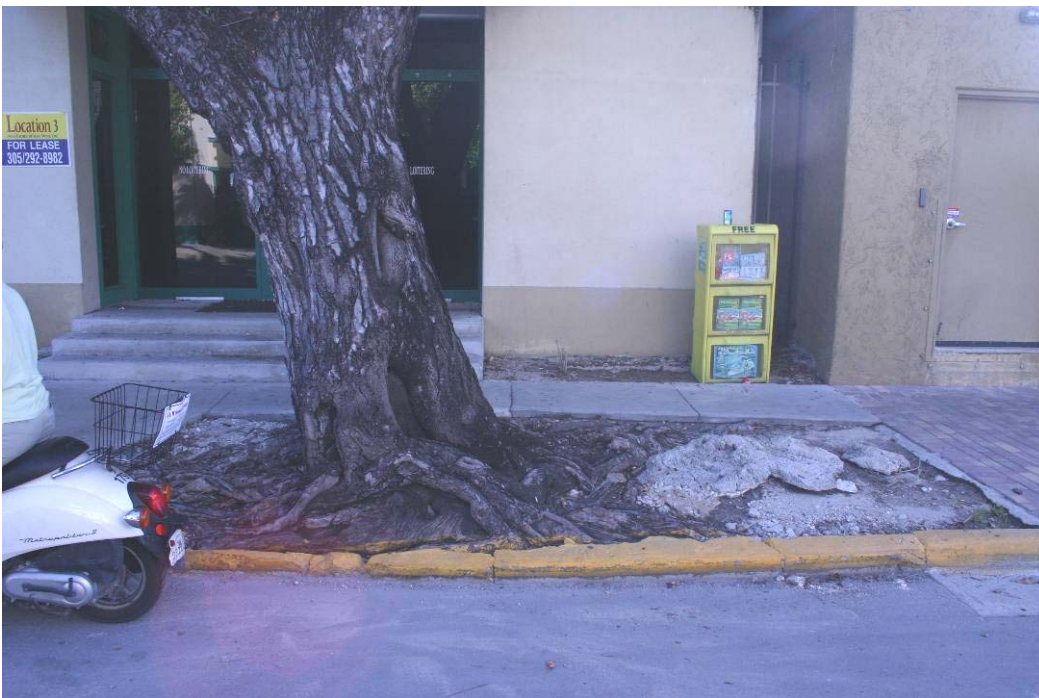
Top Photograph: Vacant Warehousing/Storage Area, Green and Simonton Street (Source: City of Key West, 2009) Bottom Photograph: Deteriorated Sidewalk, Green Street (Source: City of Key West, 2009)
