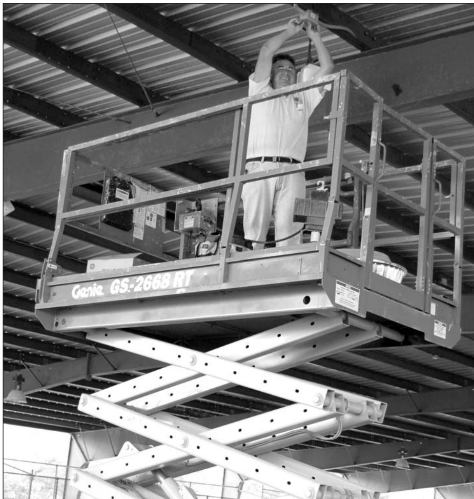
Brett Wright of the Public Works Facilities Maintenance Team works on lighting in the Key West inline hockey rink.
