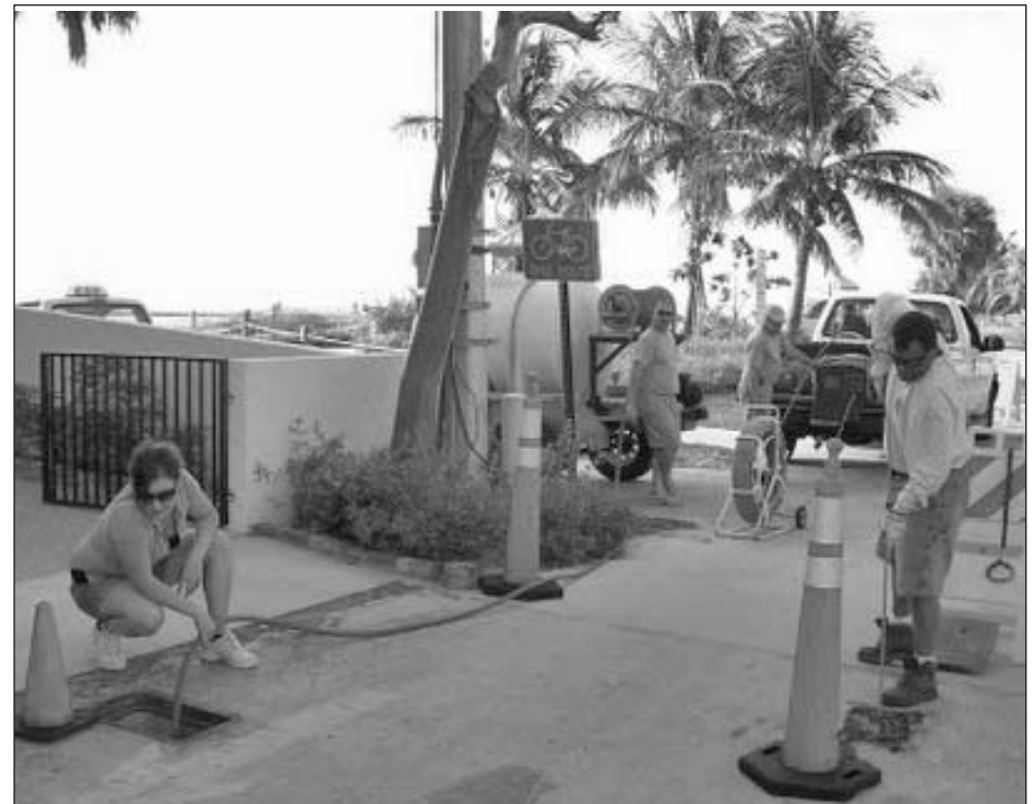
In front, Jaime Baker and Chris Hughes test a sewer lateral line while Nick Richardson and Charlie Smith look on.
