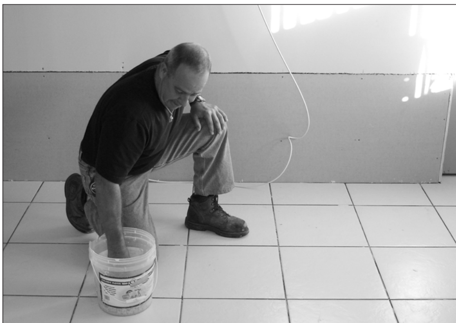
Charles Sawyer puts in new tile, repairing flood damage to Fire Station #3 on Kennedy Boulevard.
